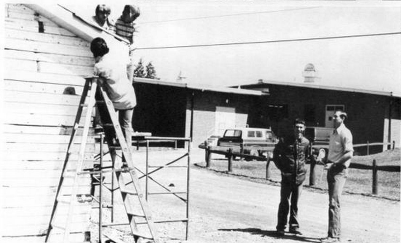
Above, Mr. Sam Taylor, Carpentry teacher, instructs his students about a building repair. Working on the building are David Walton, junior, and James Nicely, junior, and standing on the ladder is Clyde Perkins, junior. Standing with Mr. Taylor is Kevin Hefner, sophomore.
